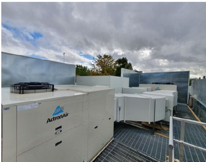
New roof top air conditioning plant
