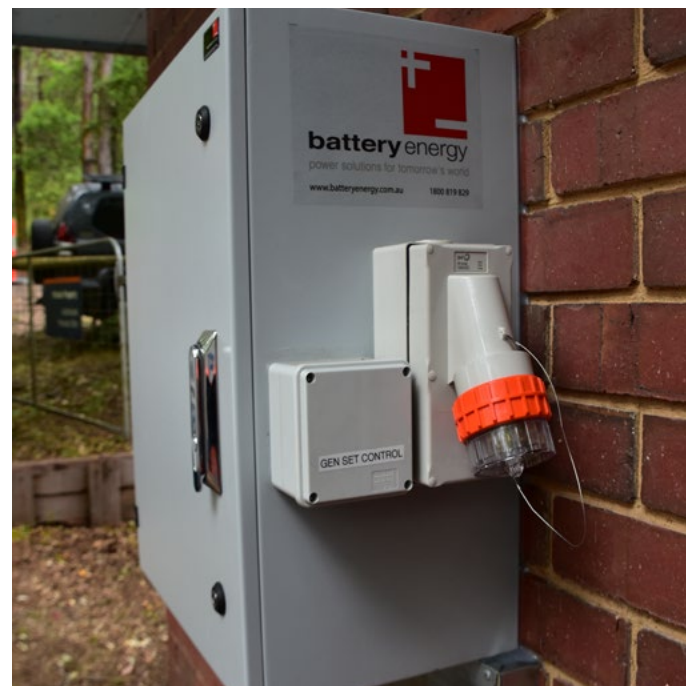
Automatic transfer unit located at Powelltown Exchange
